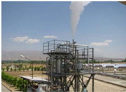
Fig. 3. A view of heat exchangers and steam generation of Shiraz solar power plant.
